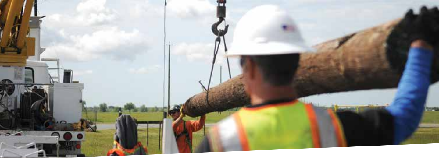
Construction workers load a power pole onto a truck to make room for its replacement at Beale Air Force Base, California. The new poles will weather storms more reliably and help meet Beale's increased energy demands. (Photo: U.S. Air Force)
